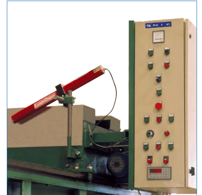
Control panel and laser beam alignment system
